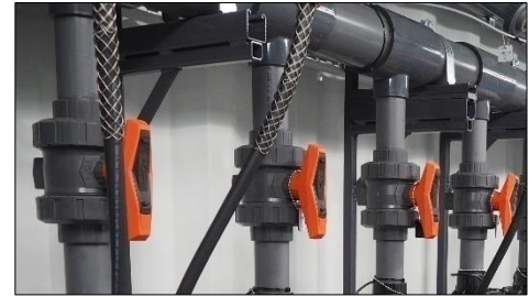
Figure 5: EC Treatment Cell Influent Isolation Valves
