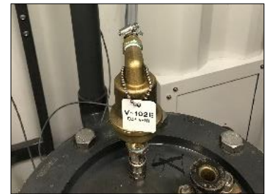
Figure 7: EC Vent Valve
