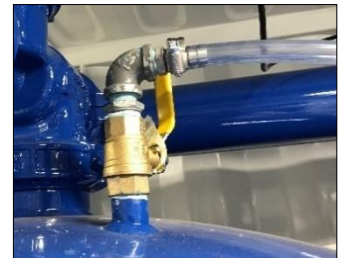
Figure 17: Media Filter Vent Valve
