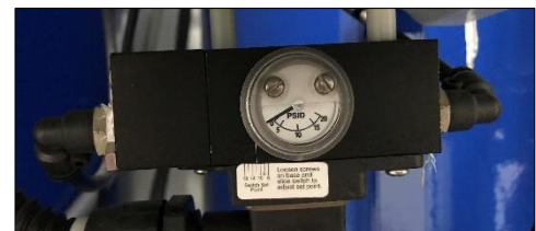
Figure 14: Media Filter Pressure Differential Indicator
