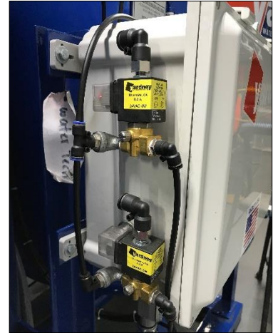
Figure 15: Media Filter Solenoid Valves
