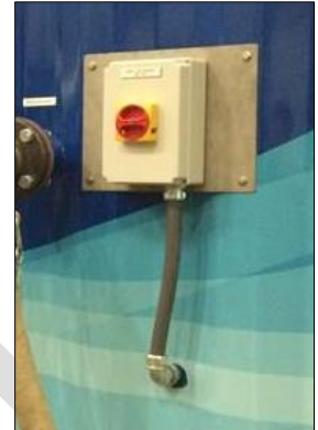
Figure 2: Source Pump Disconnect
