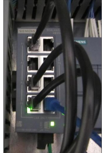
Figure 43: Unmanaged Ethernet Switch
