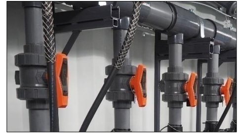
Figure 5: EC Treatment Cell Influent Isolation Valves
