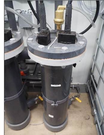
Figure 4: EC Treatment Cell
