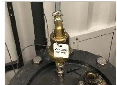
Figure 7: EC Vent Valve
