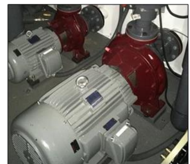
Figure 11: Media Filter Supply Pump
