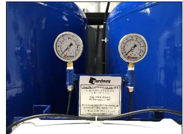
Figure 13: Media Filter Pressure Gauges
