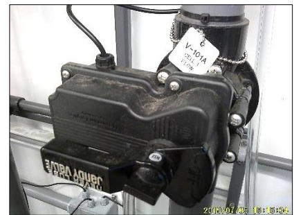
Figure 6: EC Treatment Cell Flow Valve
