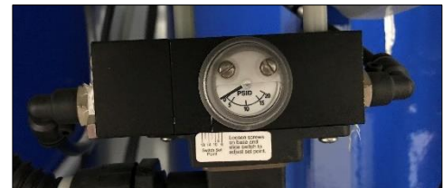
Figure 14: Media Filter Pressure Differential Indicator
