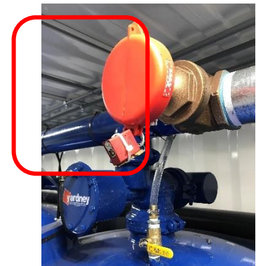
Figure 19: Media Filter Backflush Restrictor Valve
