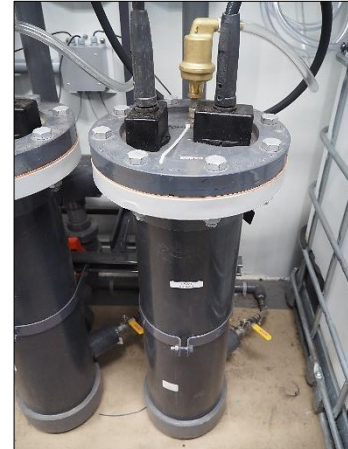
Figure 4: EC Treatment Cell
