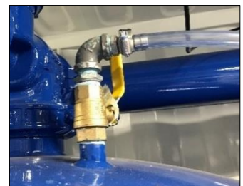
Figure 17: Media Filter Vent Valve
