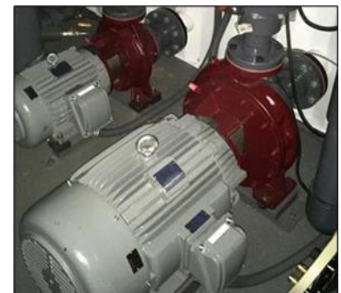
Figure 11: Media Filter Supply Pump
