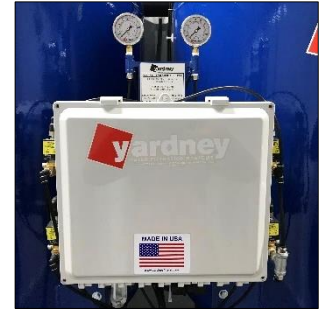
Figure 12: Media Filter Control Panel
