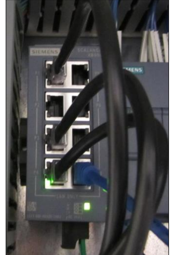
Figure 43: Unmanaged Ethernet Switch
