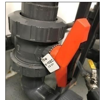
Figure 10: EC Effluent Valve
